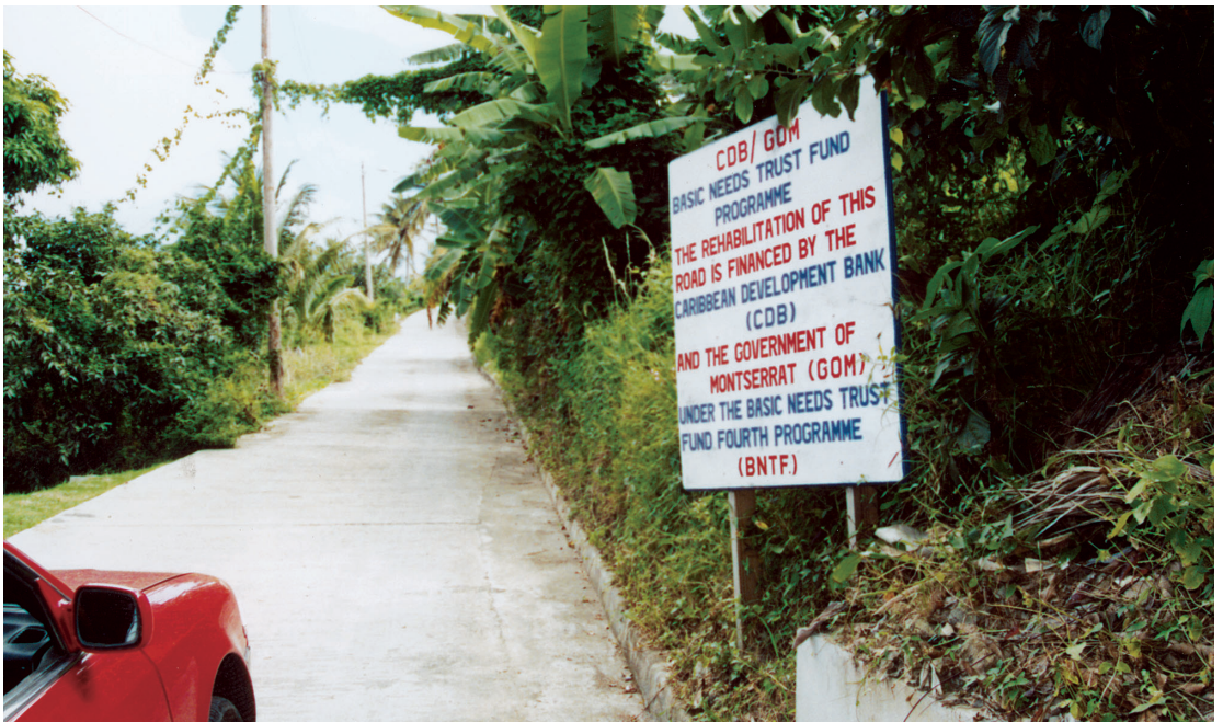
In Montserrat, a number of roads such as this one have been constructed under CDB's BNTF programme, making life a little easier and safer for the residents of the communities involved.
